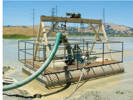
Water transfer / pumping setup
